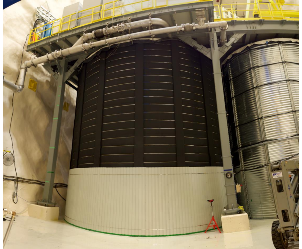
Shield Tank and emergency vent lines, tank was filled with water Oct 2015
